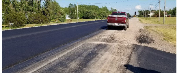
Photo 5 – Looking south (to the right) on Route 15 from Cormier Road toward Portage Road
