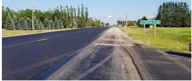
Photo 3 – Looking south (to the right) on Route 15 from the Site Access toward Cormier Road
